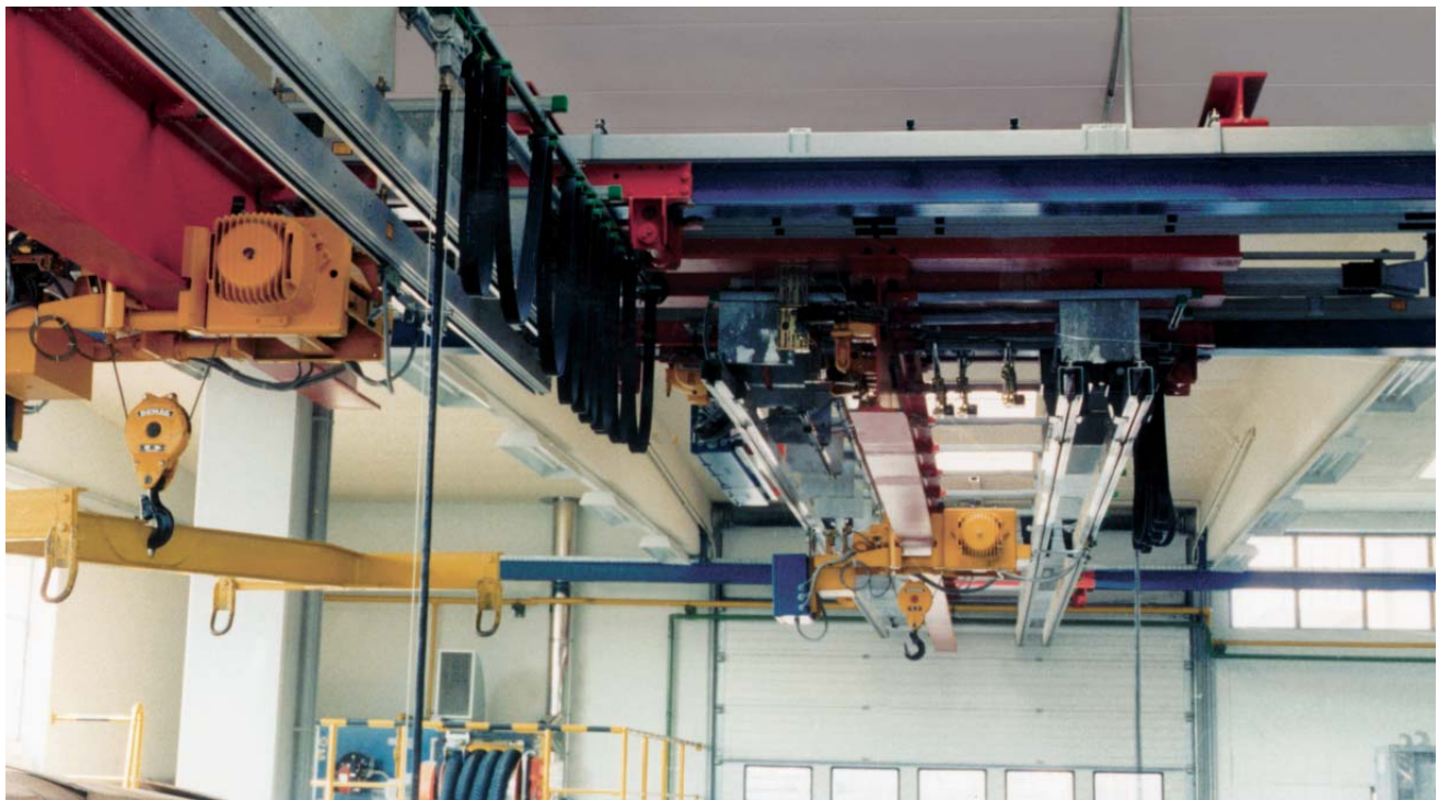
Aluminium enclosed conductor system on crane bridge.
